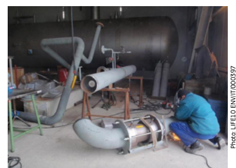
ORC-based heat recovery plant in Riesa, Germany
