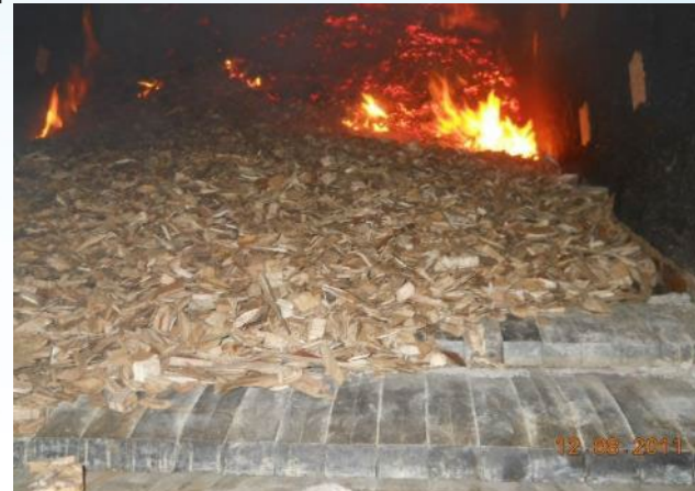
2 Biomass boilers a 10 MWh
