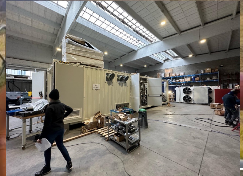
Closed loop testing unit– Storengy, GGP, MAGMA, IFPEN
