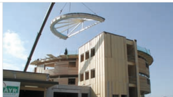
The entire wooden structure and the building's cladding were prefabricated in a workshop and assembled in only nine days.
