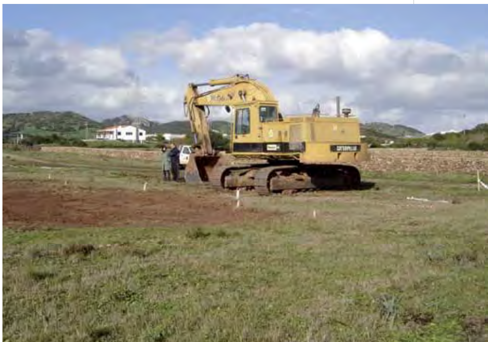
Excavation of an experimental temporary pond for educational purposes in Santa Eularieta
