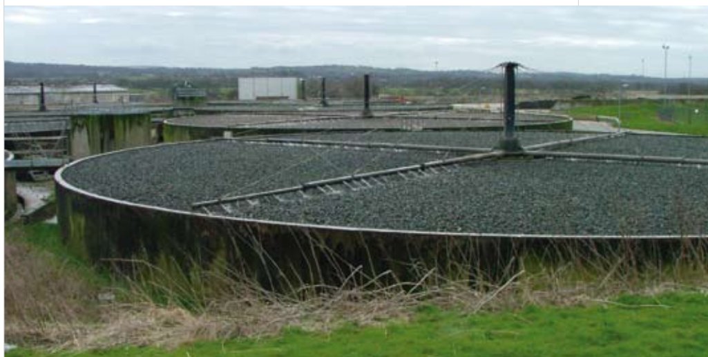
The wastewater is initially treated by traditional settling and filtration methods
