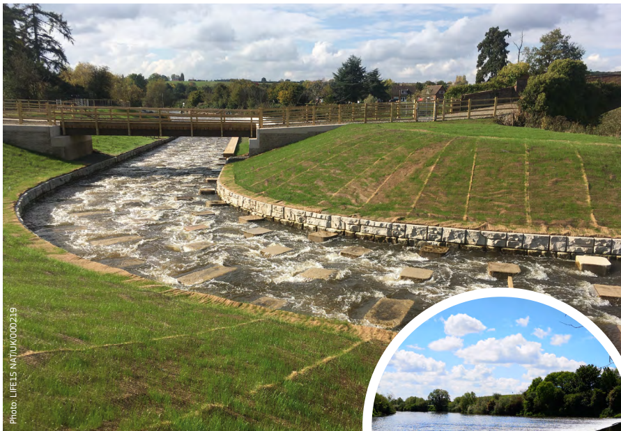
Innovative fish passes installed on the River Severn
