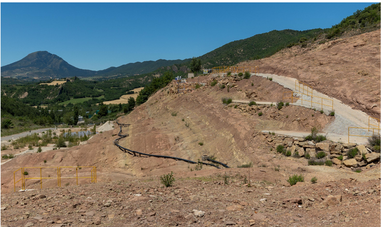
Figure 1. Old Bailin landfill (ES) in which the DISCOVERED LIFE actions have been carried out
