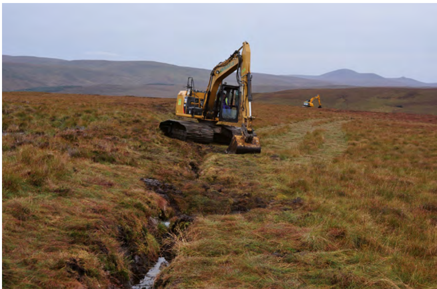
Photo: An excavator closing drainage ditches at the project site - LIFE00 NAT/UK/007075 - © Hans Joosten
