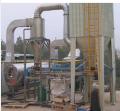
CLONIC's thermal dry pilot plant.
