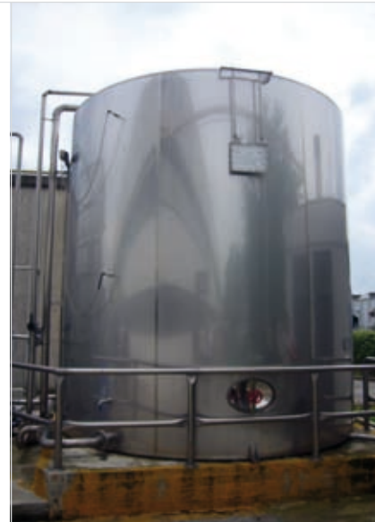
The project used a large balance tank.
