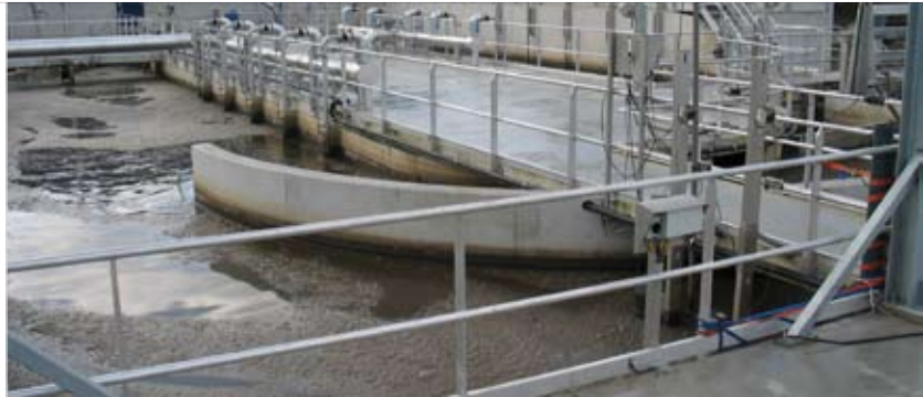
Biological purification: bacteria feed off the waste in aeration tanks
