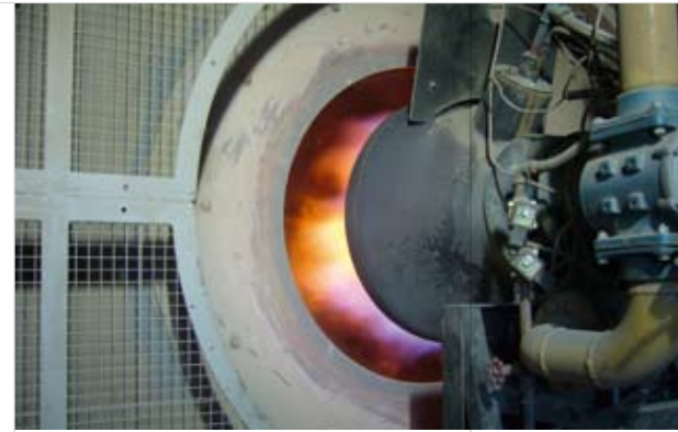
The even distribution of aggregate in the barrel means the powerful flame heats it more efficiently
