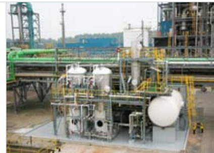
The brine recovery finishing unit was made up of salt removal columns and a carbonate destruction system
