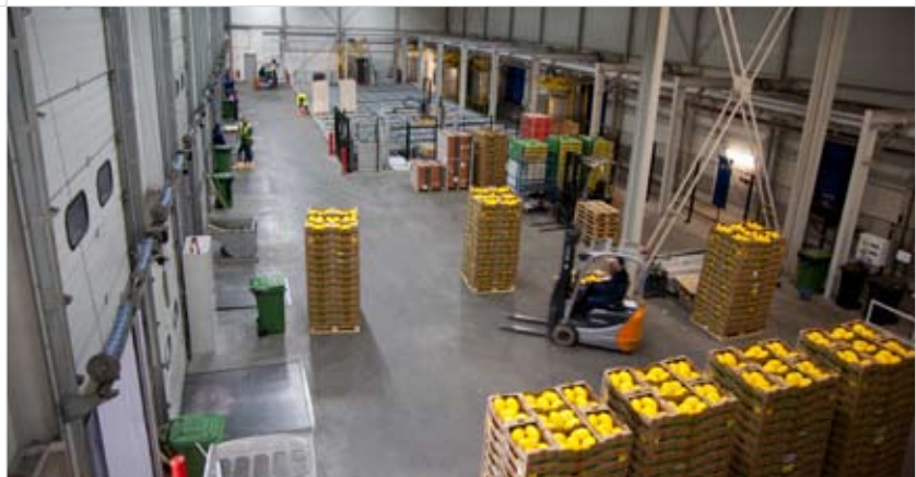
The HEIGHT project demonstrated that a high rise cold store using ammonia and CO 2 technology offers energy savings of around 75% compared with conventional cold stores
