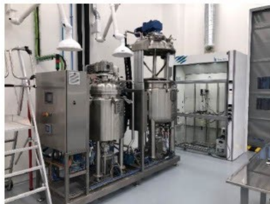
New encapsulation production line installed by Carinsa
