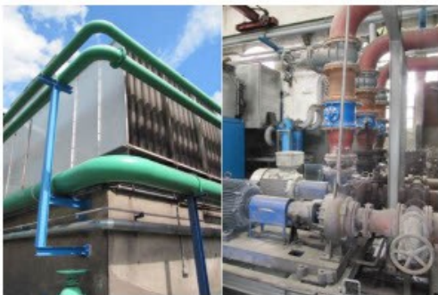
Cooling tower and water pump at Deutsche Edelstahlwerke
