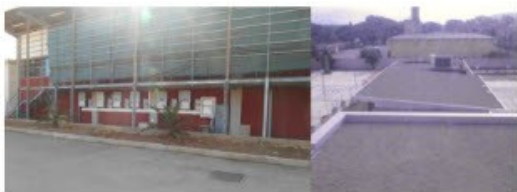
Inverters and electrical cabinets of the PV plant and new building wing with thermal insulation on the roof at Santa Maria La Palma
