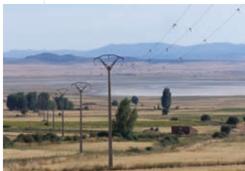
Protected electric lines
